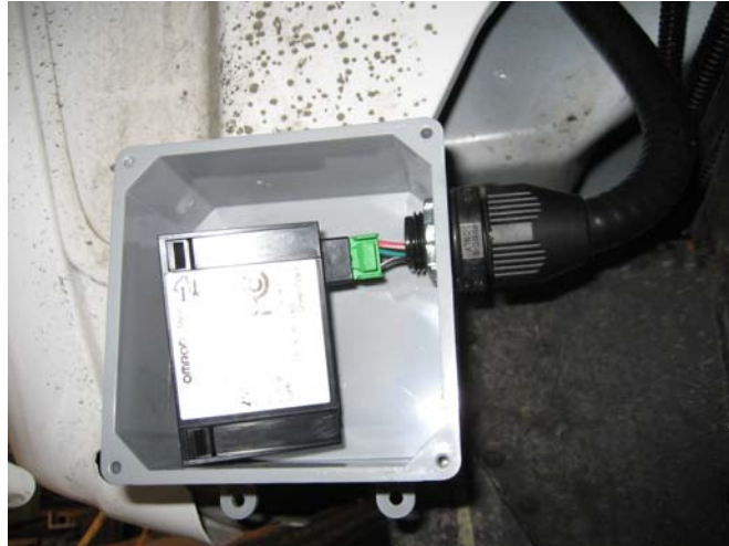
Figure 4: Mounted Enclosure w/ Module & Wiring (looking forward)
