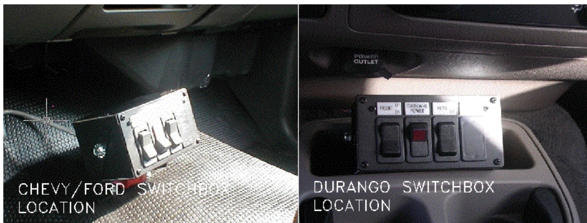
Figure 3: In-Cab Switchbox Locations
